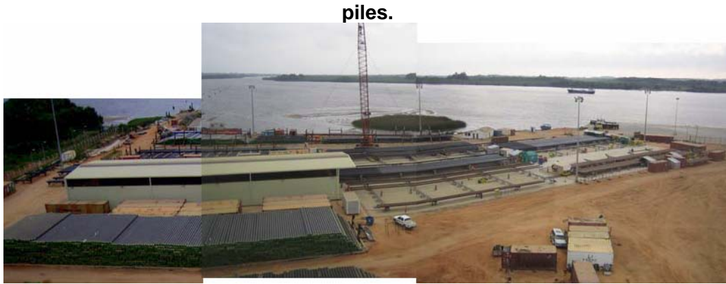
Figure 3: View of the PiP fabrication site : bare pipe quadjoint firing line front right, insulation placement in the white building, PiP insertion, welding and pressure drawdown to the far right.
